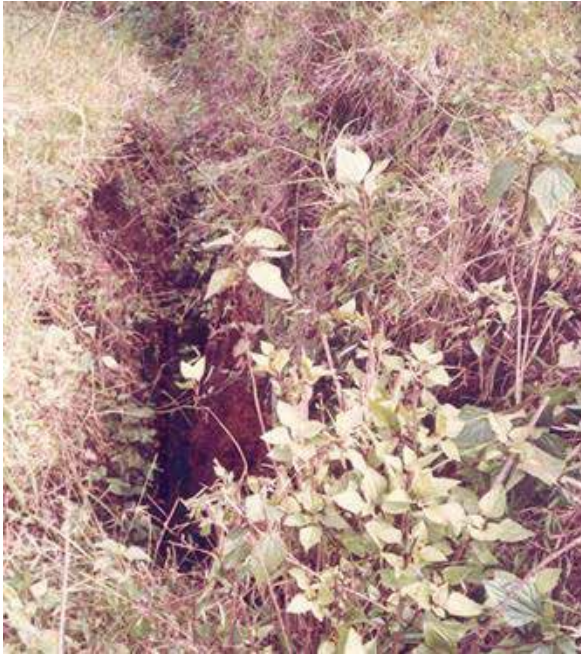
Picture 3 Perumalmalai Subsidence
