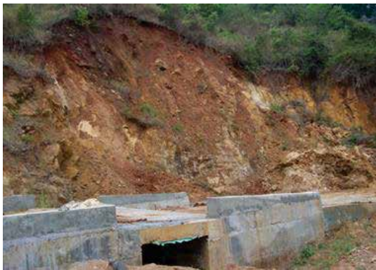
Picture 9 Alagarmadai Cutslope Slide
